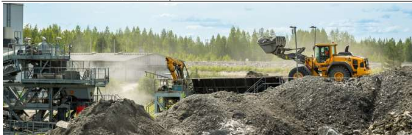
Daily operations at Endomines's Pampalo processing plant
